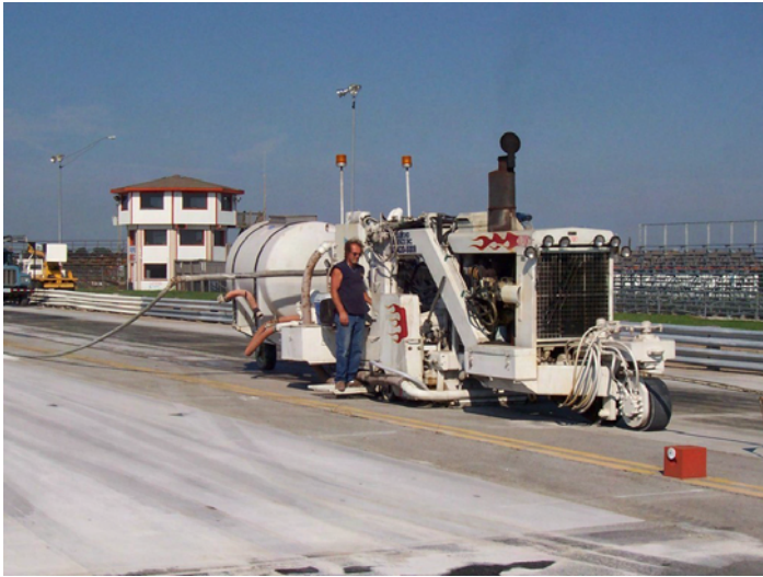
Photo is of one of Diamond Surface's long time employees grinding the Nebraska Motorplex dragstrip in Scribner, NE.
