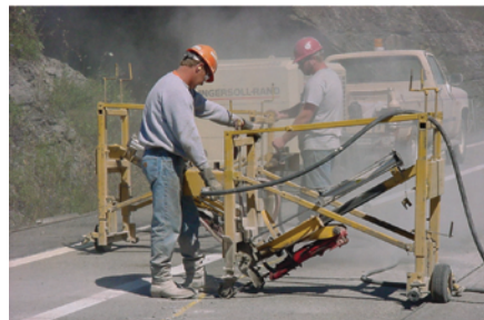
↗ 1. Drilling hole for tie bar along longitudinal crack using frame-mounted drill rigs.
