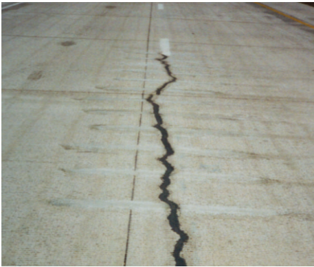
⚡ Stitched longitudinal joint and crack.
