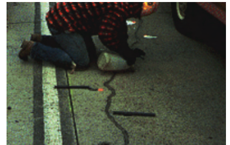
↗ 4. Pouring epoxy into drilled holes. (Injecting epoxy is preferable for large quantities.)
