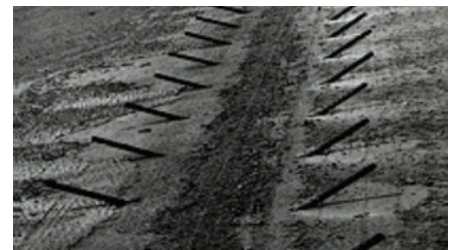
↗ 5. Inserting bars into prepared holes containing epoxy. (Note: The bars shown here are in position but not fully inserted.)
